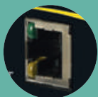
IEC 61850 server Ethernet port
