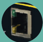
IEC 61850 server Ethernet port
