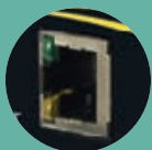
IEC 61850 server Ethernet port
